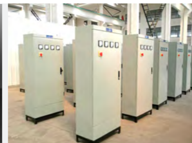
MANUFACTURING AND PAINTING OF ELECTRICAL CABINETS
