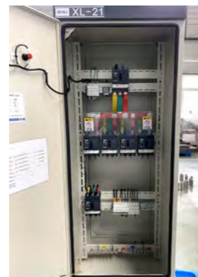
Inside of Power Cabinet
